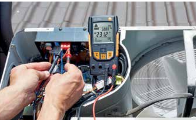
Measuring voltage on an outside refrigeration unit with testo 760 .
