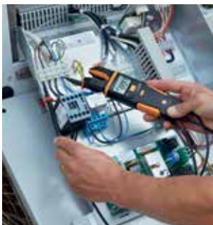
Measuring voltage on a compressor.
