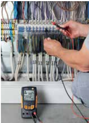
Testing voltage in a switching cabinet.
